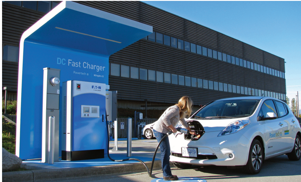
Customer fueling at Powertech's direct current fast charging (DCFC) station
